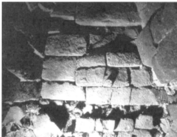
Photo 1 Falling and sliding of the front wall of the burial chamber (measured using reflected light)
