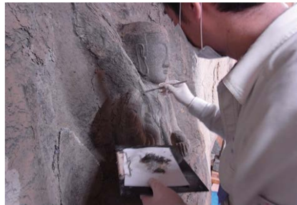
Applying epoxy resin to the cracked part, then creating a stone texture that blends with the surrounding areas
