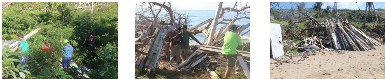
Team lifting the timbers from the site to the beach front; team stacking the timbers according to their sizes and extracting nails. Images credit: Fiji Museum
