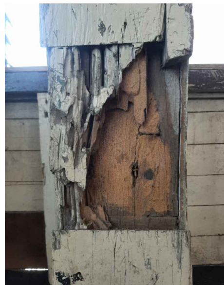
Figure 1. A wooden post in the Old Convent of Manaoag Church showing damage and loss of material. (Photo courtesy of Escuela Taller de Filipinas Foundation, Inc.)
