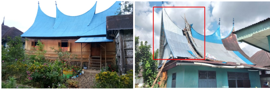
Picture 5. Bagonjong roof that is supposed to be smoothly curving. Source: PDA, 2018
