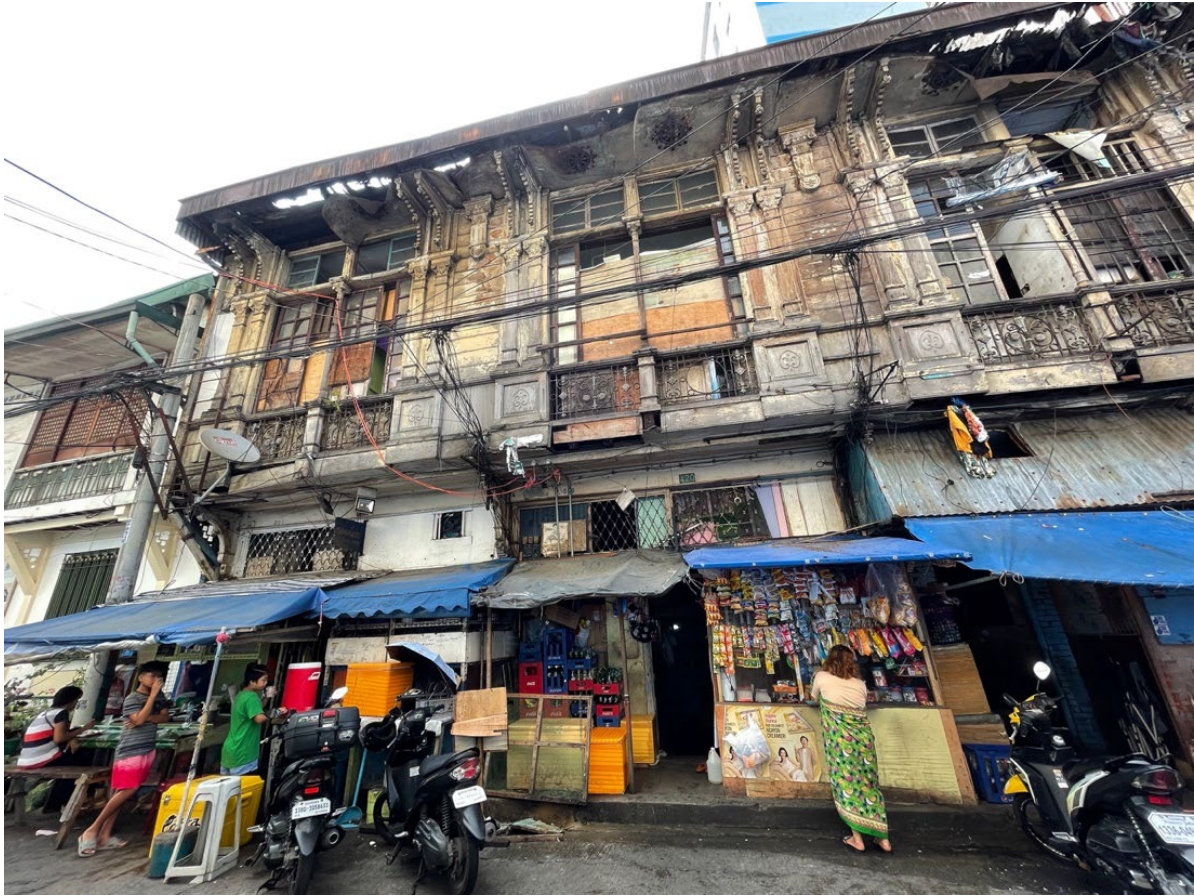
The Boix House in poor condition with informal tenants in Bautista St.
