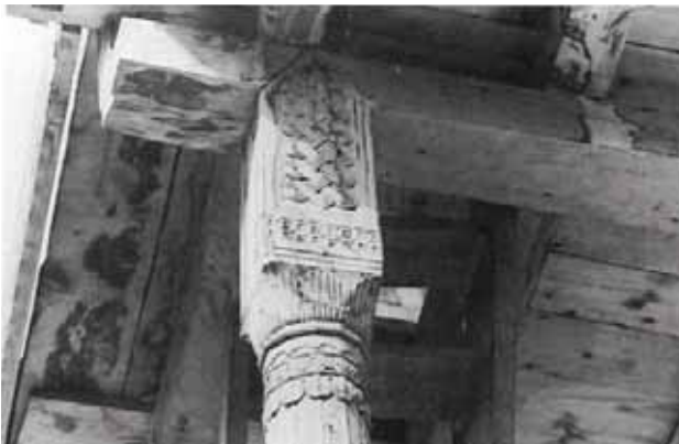
FIGURE 2. A wooden pillar and column in a dilapidated condition due to weather effects
