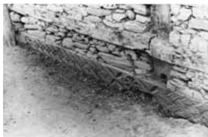
FIGURE 4. Old wooden base of wall showing deteriorated condition
