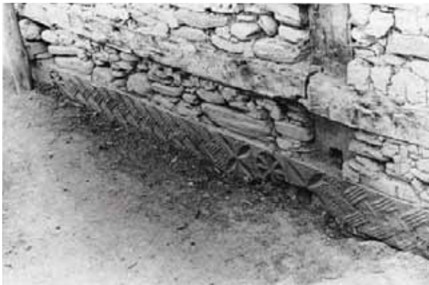
FIGURE 1. The wooden base of a wall showing its deteriorated condition due to weather effects
