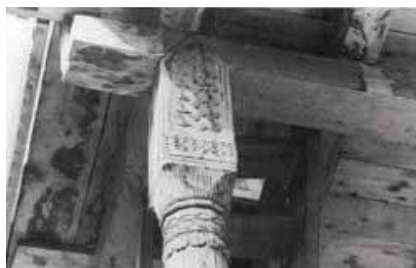
FIGURE 5. Wooden pillar and column in dilapidated condition
