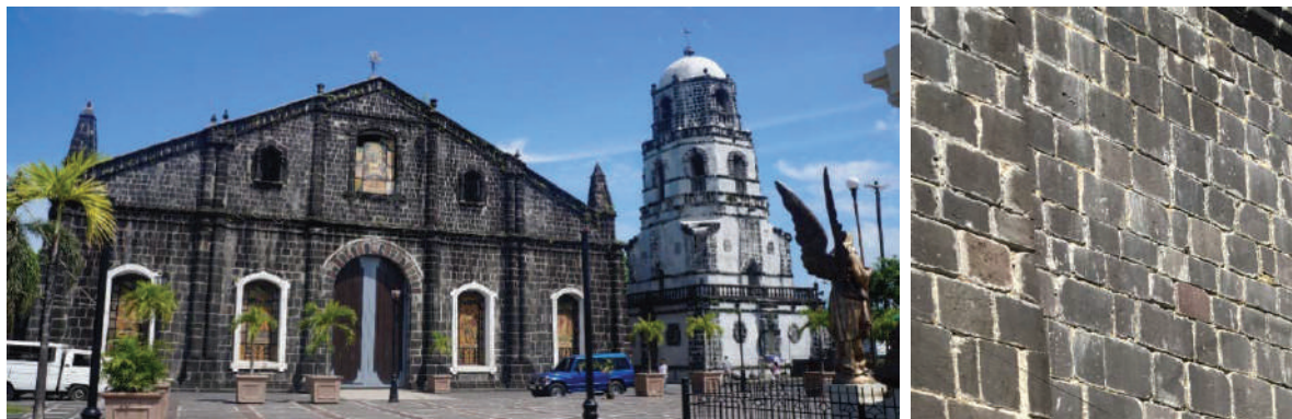
Fig.5 (left) Pre-restoration façade of the Tabaco Church, featuring hewn dark volcanic stones, NHCP, 2017
