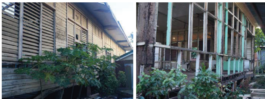
Fig.8–9 Dilapidated wooden components of Sorsogon East Central School FIGoogle photos, 2017
