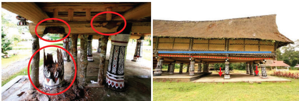
Fig.5 Material and structural damage in the Bolon House
