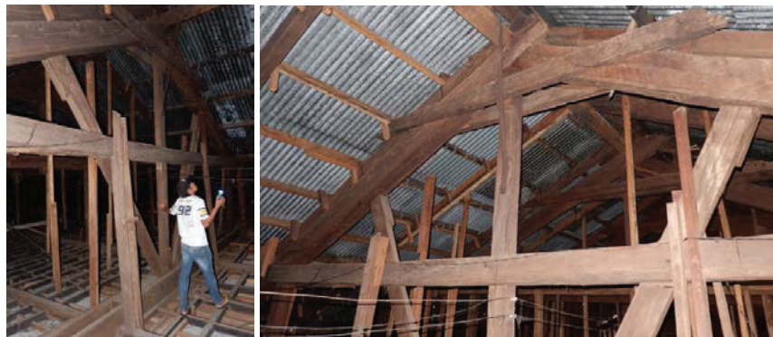
Fig.3–4 Photos of Tabaco Church original timber trusses supporting the ceiling and wooden framing, Arch. Lorilla, 2018 August
