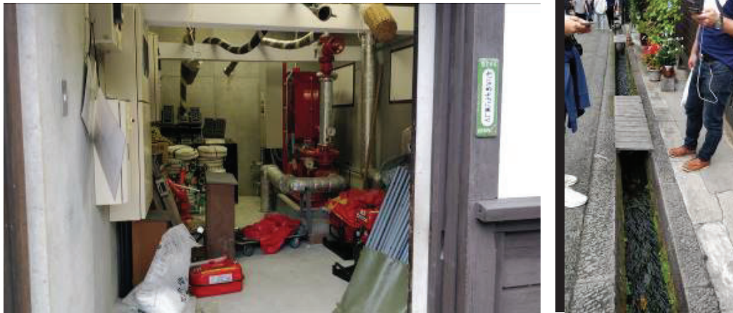
Firefighting implements and drain in Takayama city
