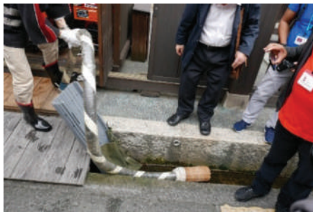
Fig.1 Fire protection system in Takayama city
