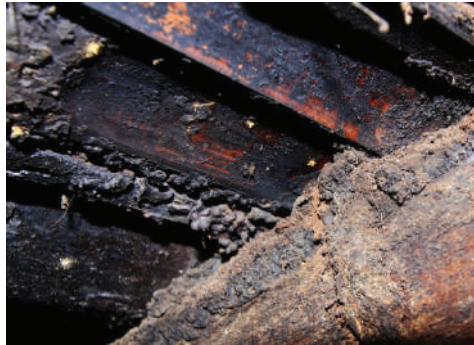
Fig.6 Layer of soot on the beam above the kitchen
