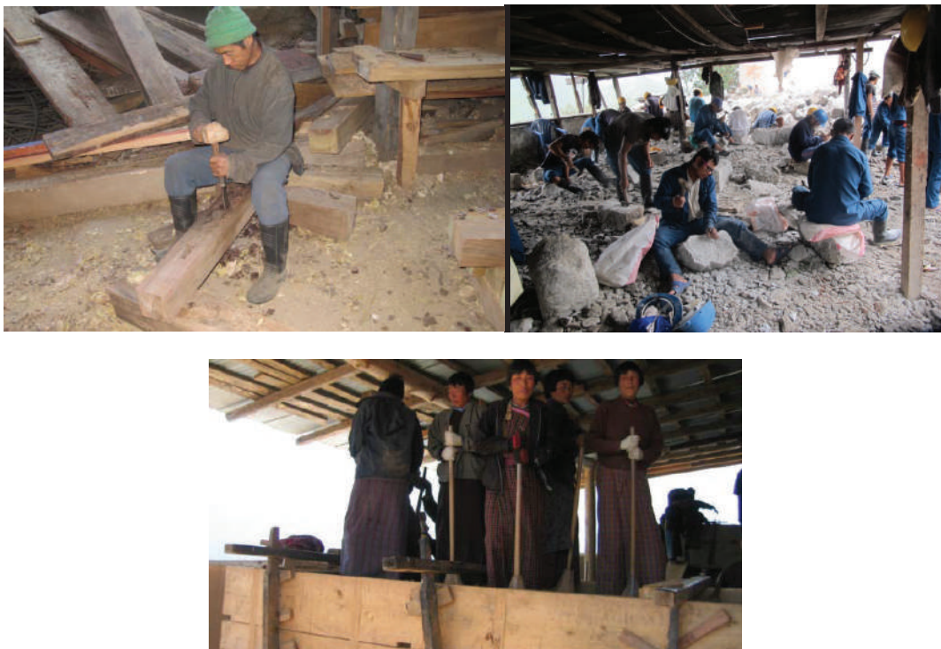
Fig.2 Carpenter working on traditional joinery detail (top left); masons dressing stone (top right); women ramming earth (above)
