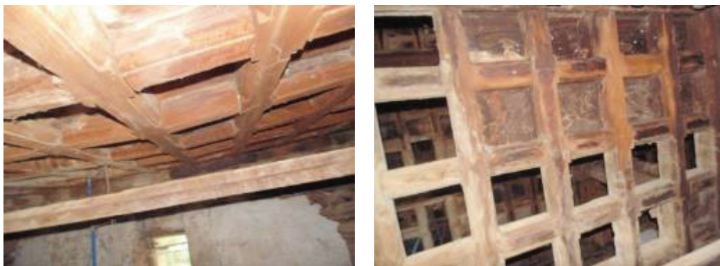
Figure 3. Timber ceiling components showing excess vertical deflection and missing panels
