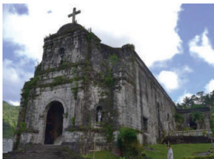
Fig.1 Pre-restoration photograph of St. John the Baptist Parish Church façade, NHCP, March 2017
