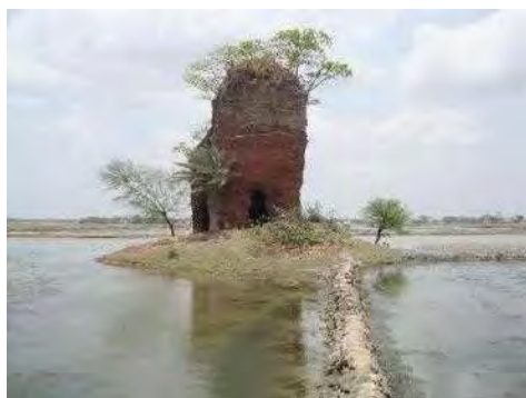
Fig.4: Erosion due to flooding, Damril Nabaratna Temple, Satkhira
