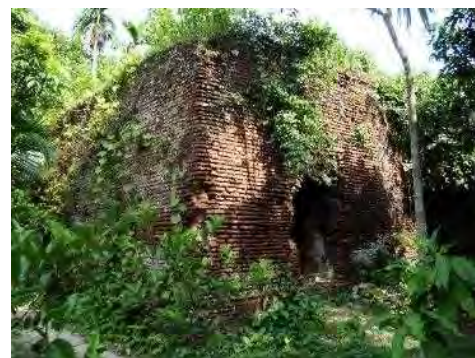
Fig.5: The effect of salinity on a building, Saroshsoti Atchji Bari, Satkhira
