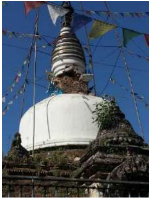
Fig7: Chilanco stupa damaged during earthquake 2015
