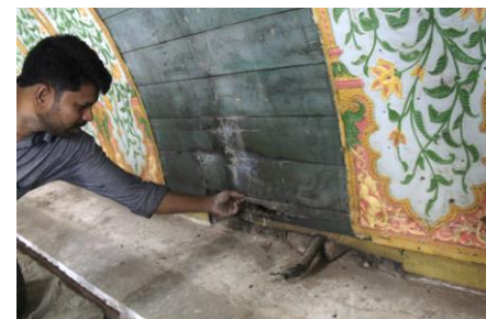
Deteriorated wooden panels supporting papier mache ceiling
