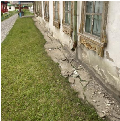
Pic 6. Rain water pipe with no drainage system
