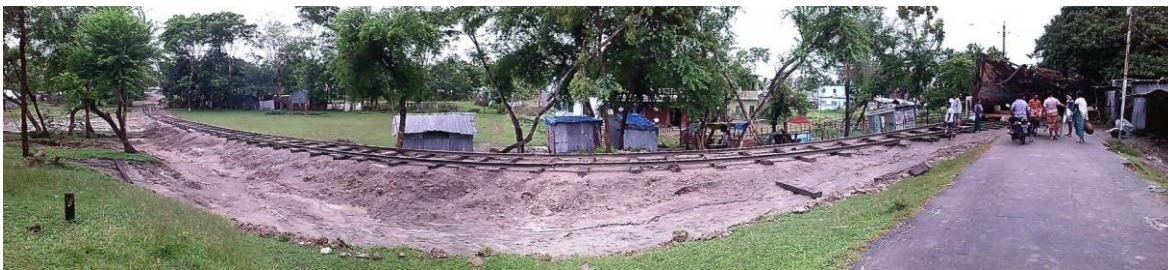
Figure 2: After excavation the 'schooner' is transported by a temporarily constructed railway line.
