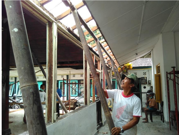
Picture 1. a senior staff demonstrated how to replace girders by lifting the roof Source: Regional Office for Cultural Properties Preservation, 2016
