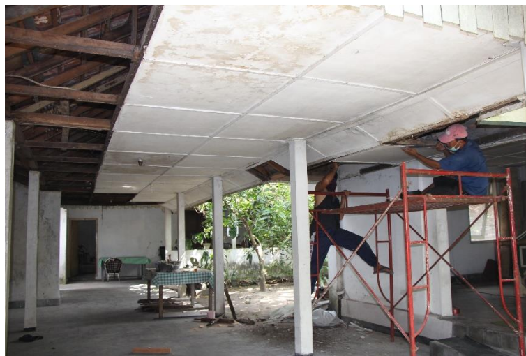
Picture 1. a senior (carpenter) worked together with a junior staff for replacing ceiling braces Source: Regional Office for Cultural Properties Preservation, 2016
