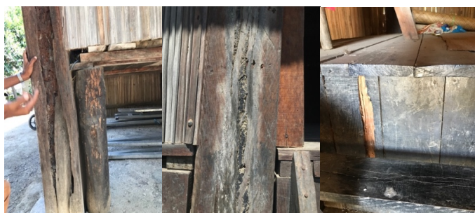
Figure 4 The condition of uma lulik of Leobesi Karketu Mota Ain: The Column that partially destroyed; The collagen of cement to the column; Partly structure that were painted by the oleo; Source: SEAC, 2023; .
