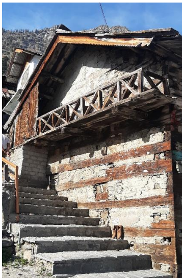
Figure 6 The side elevation of a traditional Koti Banal structure with the horizontal wooden beams and stone infill
