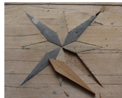
Earlier repairs – Wooden piece painted black to replace original colored wood
