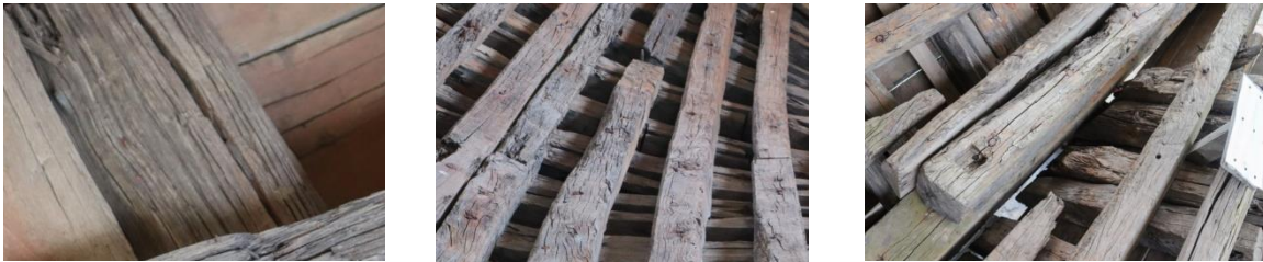
Figure 3: Cracks in wood caused by exposure to storage prior to conservation
