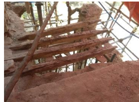
Rotten wooden joists
