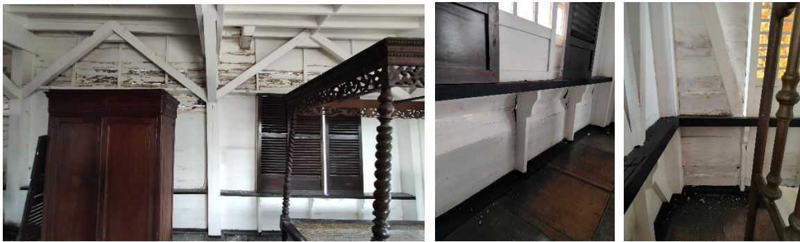
Picture 10-12: Deteriorated wooden components at one of the rooms of at the tower of Emilio Aguinaldo Shrine.
