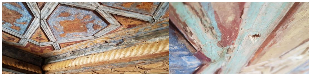
Picture 9 and 10: Holes and damage caused by pest activity (source: Meidan Emam World Heritage Office Archive)
