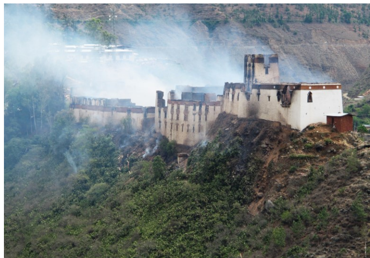
Figure 3. Dzong after fire of June 24,2012 Source: DCHS
