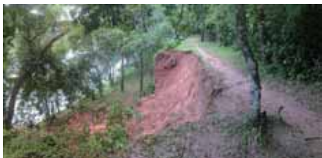
Collapsed wall in 15 m length on 13 Oct. 2011
