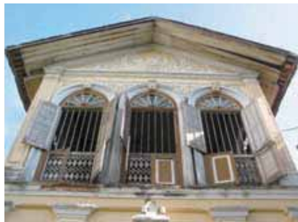
A dilapidation survey conducted on the Teh Bunga House, prior to restoration works, diagnosed serious problems affecting the building exterior and interior
