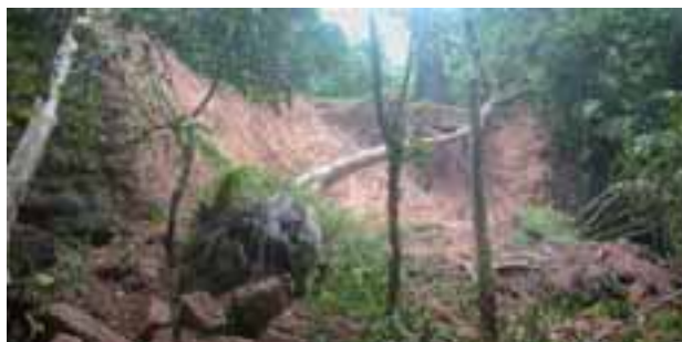
Collapsed wall in 18 m length on 14 Oct. 2011
