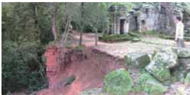
Collapsed wall in 5 m length on 15 Oct. 2011
