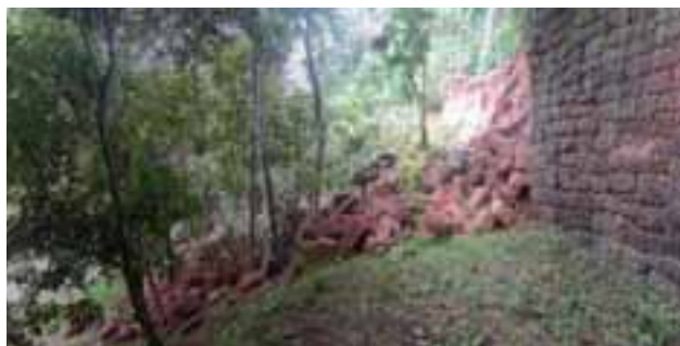
Collapsed wall in 17 m length on 11 Oct. 2011
