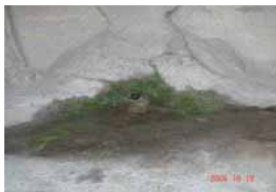
Fig. 4. Biological deterioration on the ground caused by drip water from the roof of the Yaofang Cave
