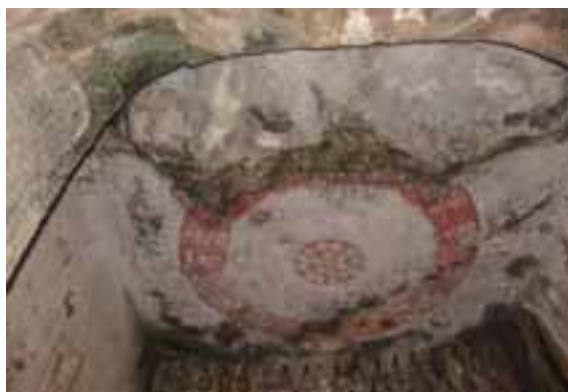
Fig. 1. Leaking water on the roof of the Wanfo Cave
