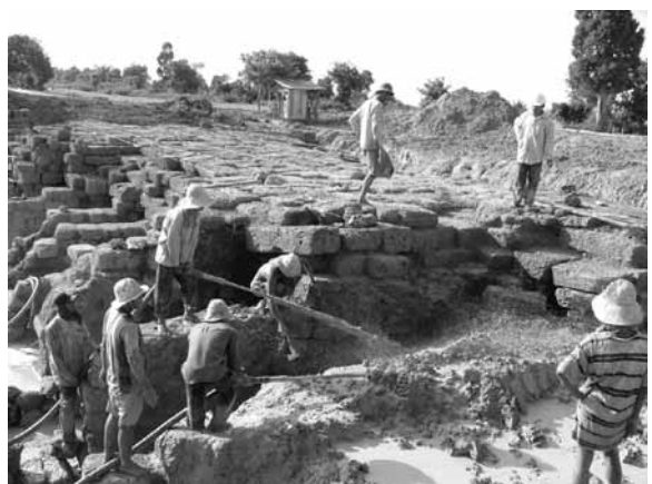
Using water pumps to wash out the soil blockages in all drainage areas
