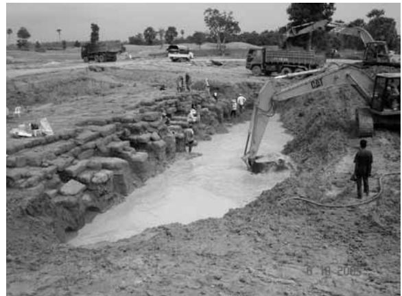
Using an excavator to clean the accumulated soil out of the bridge foot, in the aim of finding the bridge pavement and its embankment step
