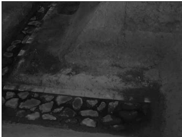
Figure 5: Mould growth on remains at the Excavation Site Exhibition Hall, Heijo Palace site Photo: Jo Wylie, Oct 3 2006
