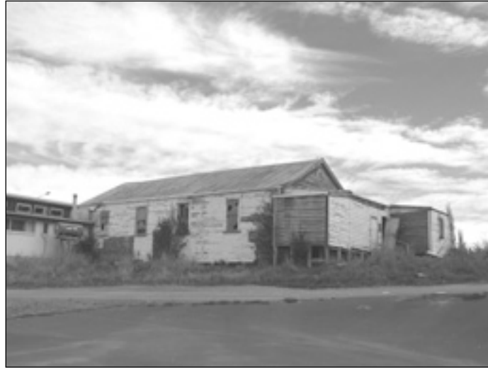
Figure 39. Waikouiti Public Hall near Dunedin, built in 1872. An example of ‘demolition through neglect’. Early social buildings such as this are often left to degrade in New Zealand and are eventually demolished, even though they represent a significant part of the local heritage and their architecture and setting is found no-where else in the world.
