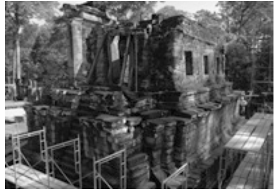
Pl. 6 Southern Library before restoration
