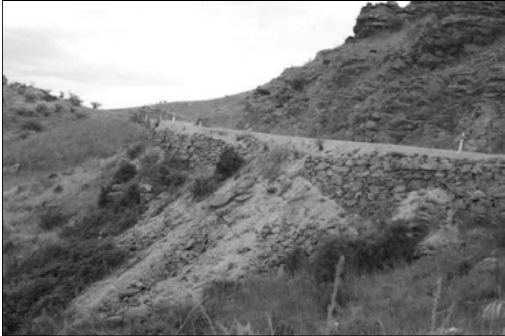
Figure 31. Stone riveting on the 1860s Old Dunstan Road, Central Otago. (photo: Matthew Schmidt).
