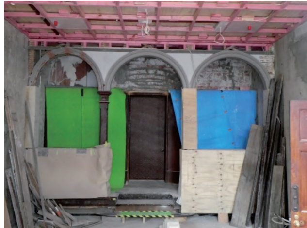
Figure 7. Former Municipal Council Chambers, showing altered library arches and new shear wall. Photograph: Gareth Wright, November 2023.
