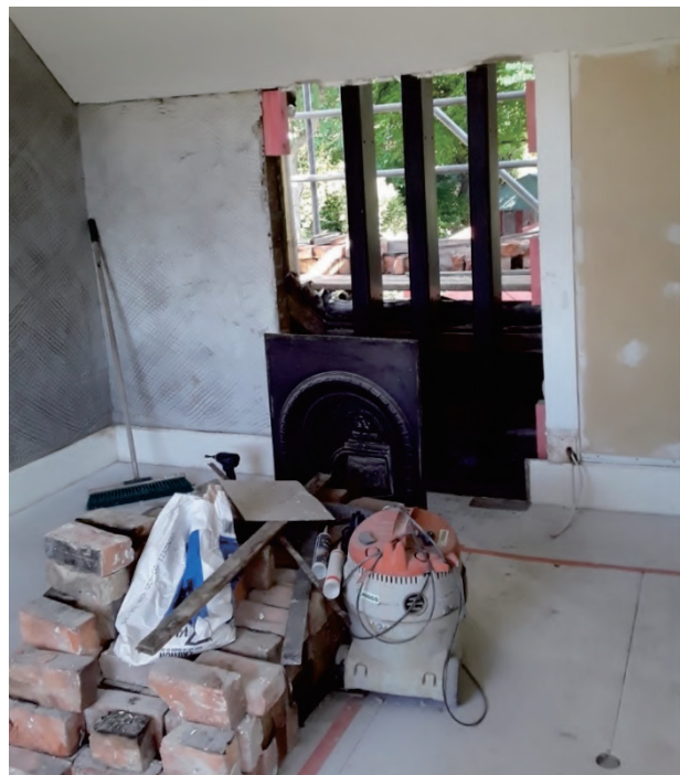
Figure 5. Former Belfast School Masters House, new steel structural chimney frame and salvaged bricks. Photograph: CCC collection.
