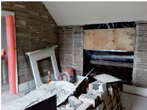
Figure 4. Former Belfast School Masters House, Exposed traditional lath structure. Photograph: CCC collection.
