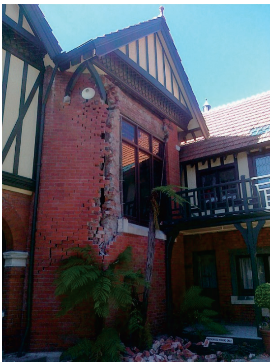
Figure 8. Mona Vale Homestead, damage to brick exterior walls. Photograph: CCC collection
