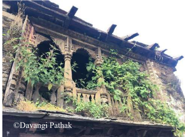
Biological growth on wooden facade known as likhai
