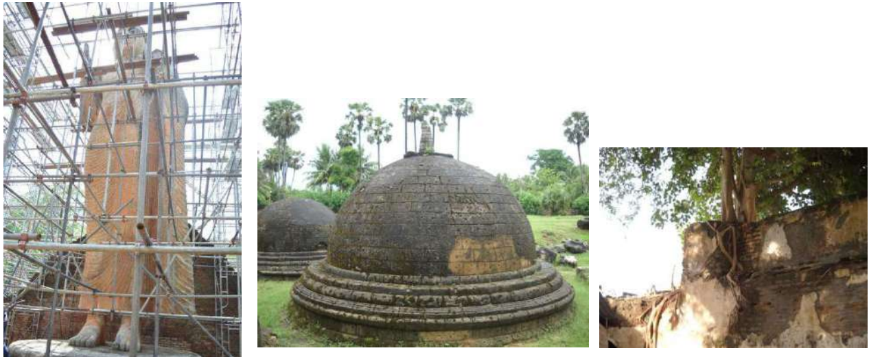
Fig. 2 Damage due to weathering
